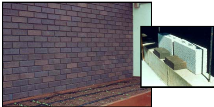
Figure 1. Brick storage wall in passive solar hobby greenhouse – Thermal storage mass is a wall made with two layers of brick filled with concrete. In this well-built structure, nighttime temperatures dropped to 35° with no supplemental heat when outside temperatures dropped to -17°. Note young crops in raised-bed style garden with drip irrigation.
