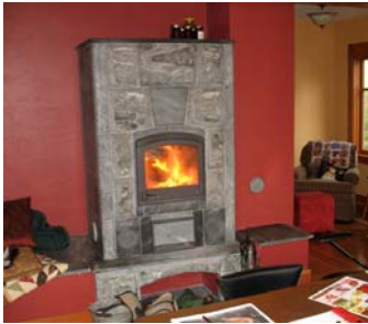
Figure 2. Photograph of Barkman family contraflow masonry heater. Pleasant Hill, Oregon.
